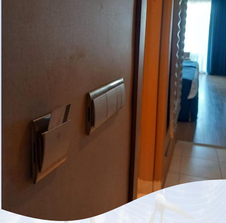
Room Energy Cards
